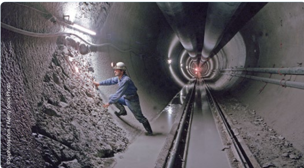
◀ An engineer examines a delivery tunnel wall on the Lesotho Highlands Water Project, which supplies water to South Africa.
